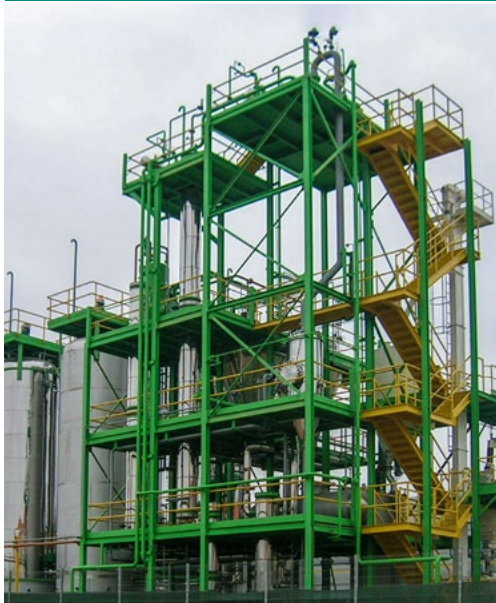
PERSEO Bioethanol® Pilot Plant
