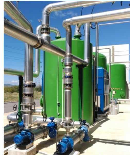
CLAMBER Pilot Plant
