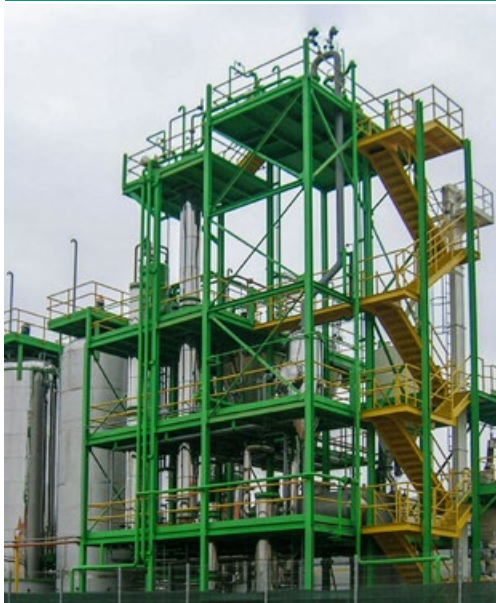
PERSEO Bioethanol® Pilot Plant
